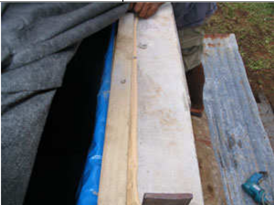
Both liners – cream outer one and blue inner one installed and secured
