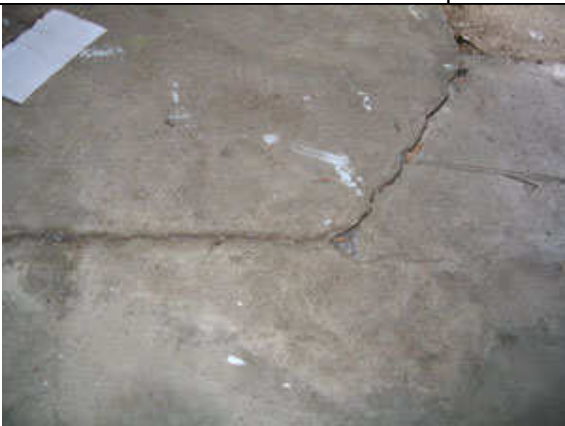
The floor slab rolled, cracked and lifted in places. It looks far worse than it is.
