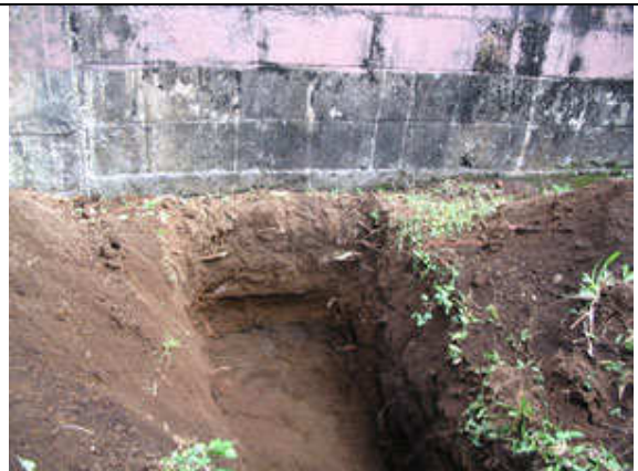
Phil organized a test trench by the affected wall – which shows the school is built on solid ground
