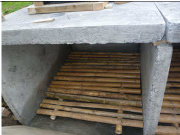
The bamboo floor of the tank 100mm off the floor. This is covered in grass and keeps the solids off the floor allowing the liquid to drain. Marine ply doors were constructed as the end wall
