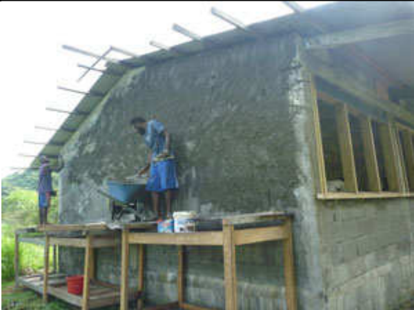
The far end wall – with exposed untreated purlins. These were later cut off and the iron flashed.
