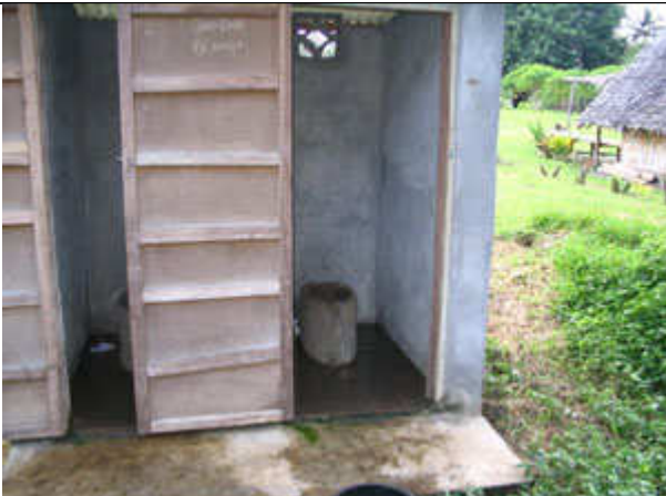
School toilets. Squat style over a septic tank
