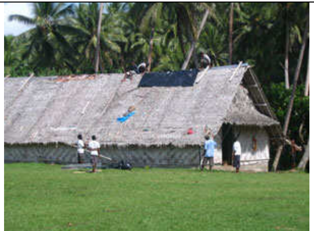
The boys' dormitory that is in need of replacement
