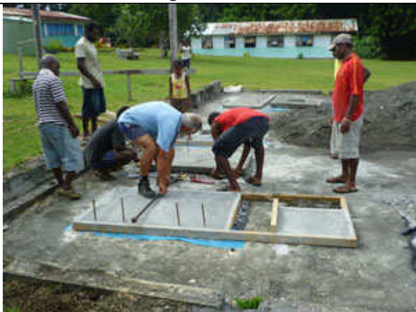
Four days later Kerry turns up to start supervising the moving of the slabs
