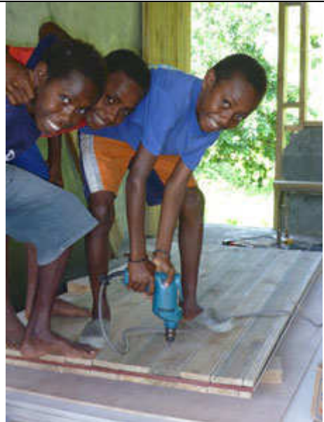
Door construction – and introducing the local kids to an electric drill and putting them to work
