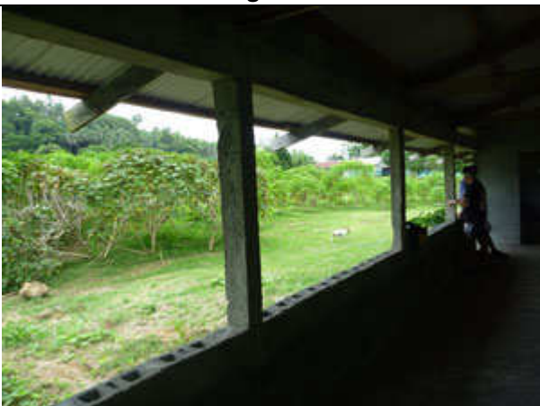
Poor column/roof support
