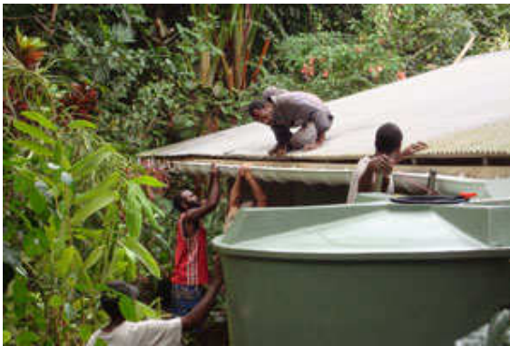
A length of 4 x 2 as a barge board and gutter brackets installed at 500mm centres
