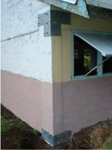
Metal plates attached in damaged areas
