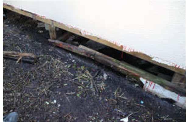
The rotten timber. The boys replaced this timber then covered it all up with fibrolite.
